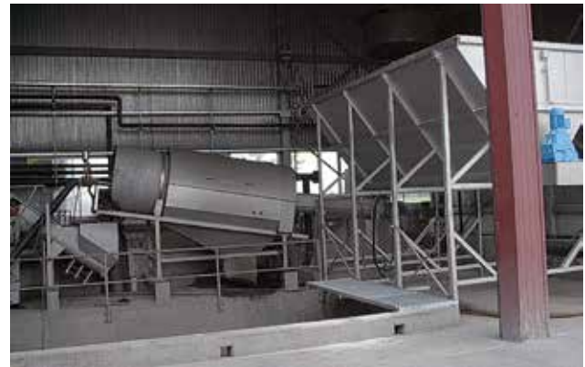
Grit acceptance area at Bolliger company (Switzerland).
