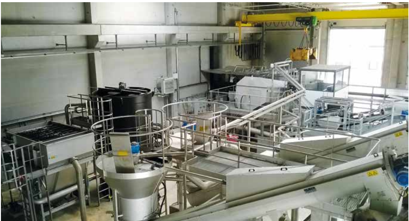
HUER Grit Treatment Plant RoSF5 Malezieux, France.
