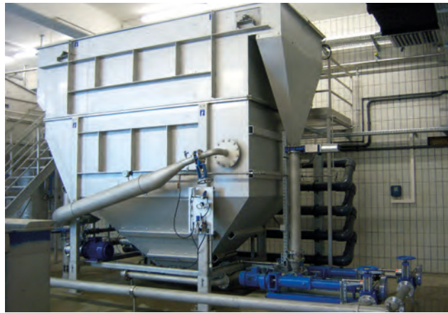
HUBER Dissolved Air Flotation for physical-chemical pre-treatment – optimum reduction of COD, fats and solids, more than 500 installations worldwide.
