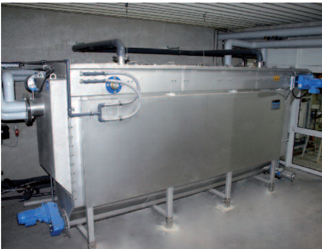
Industrial plant, 90 kW cooling capacity with simultaneous heat output of about 120 kW, used for process optimisation
