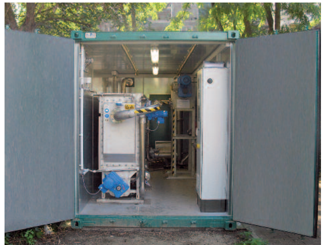
Example of a containerised solution with about 60 kW heat output used to heat a sports and day-care centre for children
