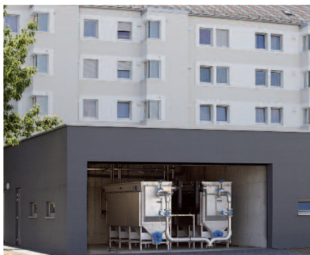
Heat station with HUBER RoWin Heat Exchanger
