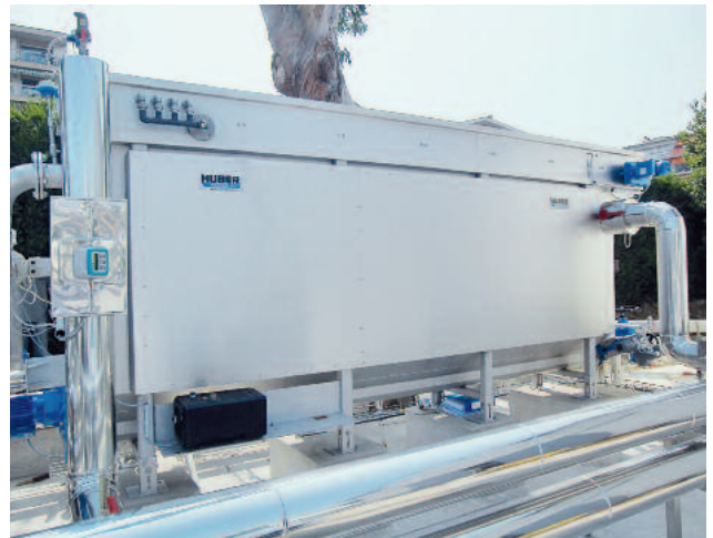
120 kW cooling capacity used to cool a storage building
