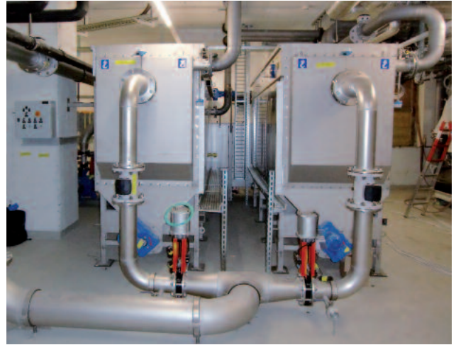
Municipal wastewater, 585 heat output, 605 kW cooling capacity, used to heat and cool an about 22.000 m 2 size office building
