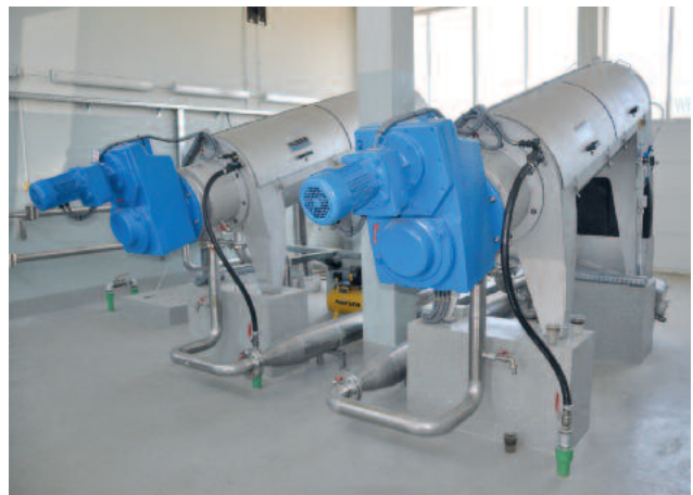
Parallel installation of two HUBER Screw Press Q-PRESS® units
