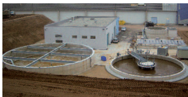
Industrial WWTP, three VRM® 30/400 units with 7,200 m 2 installed at Hans Kupfer & Sohn GmbH, Germany
