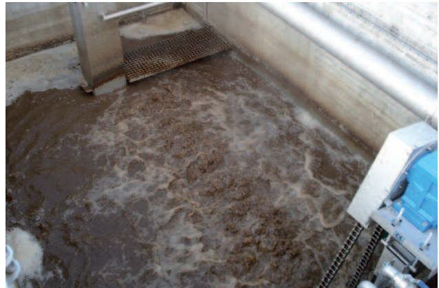
VRM® 20/300 – membrane unit installed on the industrial wastewater treatment plant GZM Lyss, Switzerland
