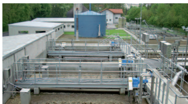
3 VRM® 30/544 membrane units installed on WWTP Hutthurm, Germany
