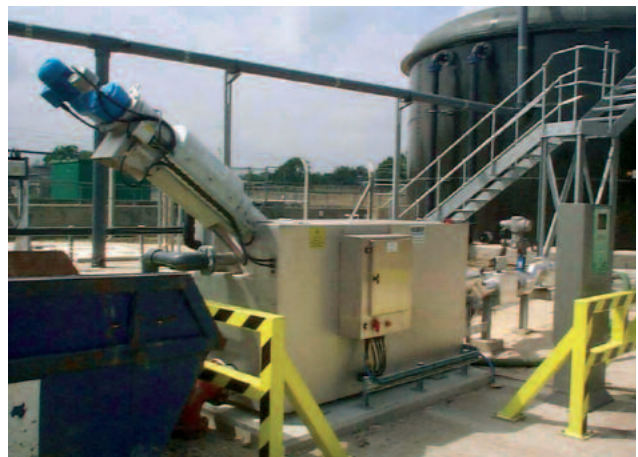
Outdoor installation of a ROTAMAT® Sludge Acceptance Plant
