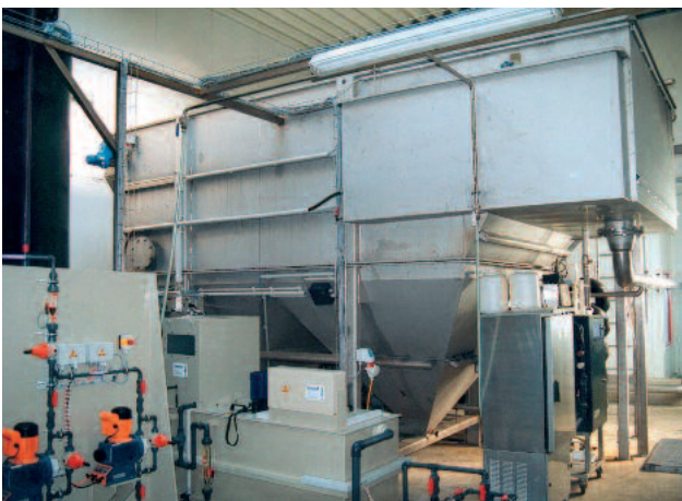
HUBER Flotation Plant HDF with chemical treatment
